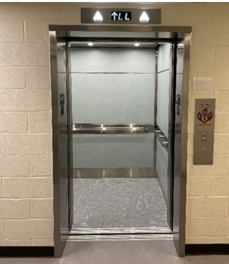
New Elevators Installed in the main hallway as well as the commissary elevator:
